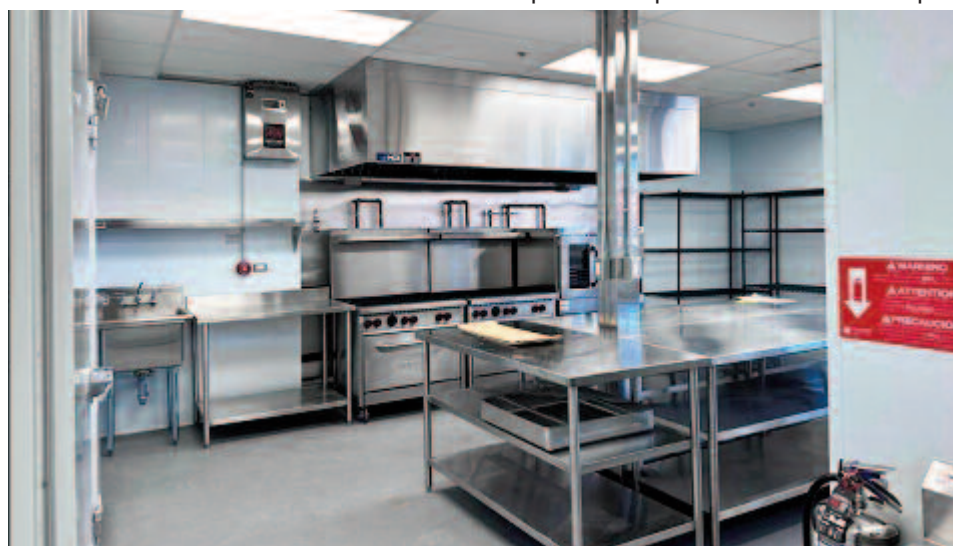
The kitchen facility being used by West Island Mission (WIM) and Volunteer West Island's Meals on Wheels program (Photo credit: Chelsea St. Pierre)
